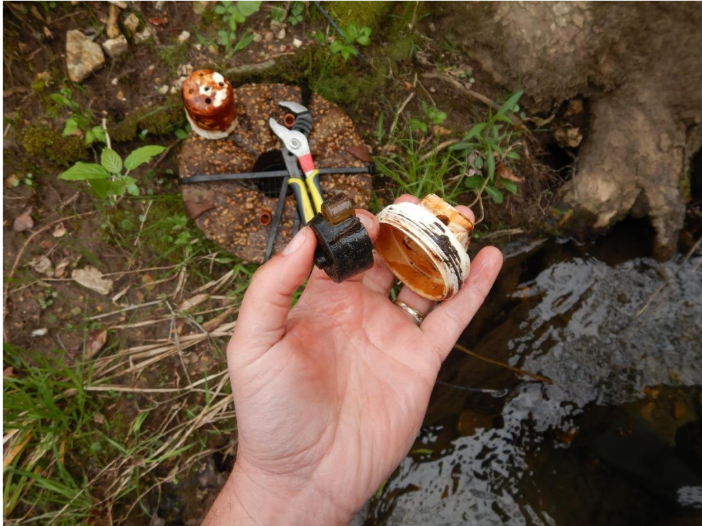
Photo 8. Temperature sensor protected by rubber boot inside PVC pipe (April 14, 2021).
