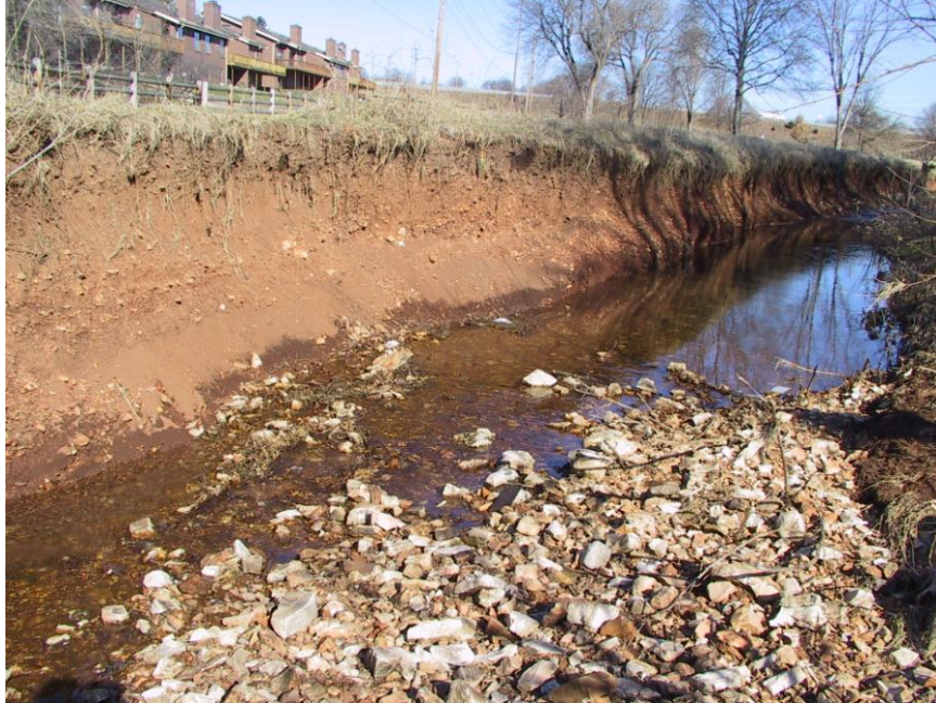
Photo 3. High bank at station 1,000 feet
