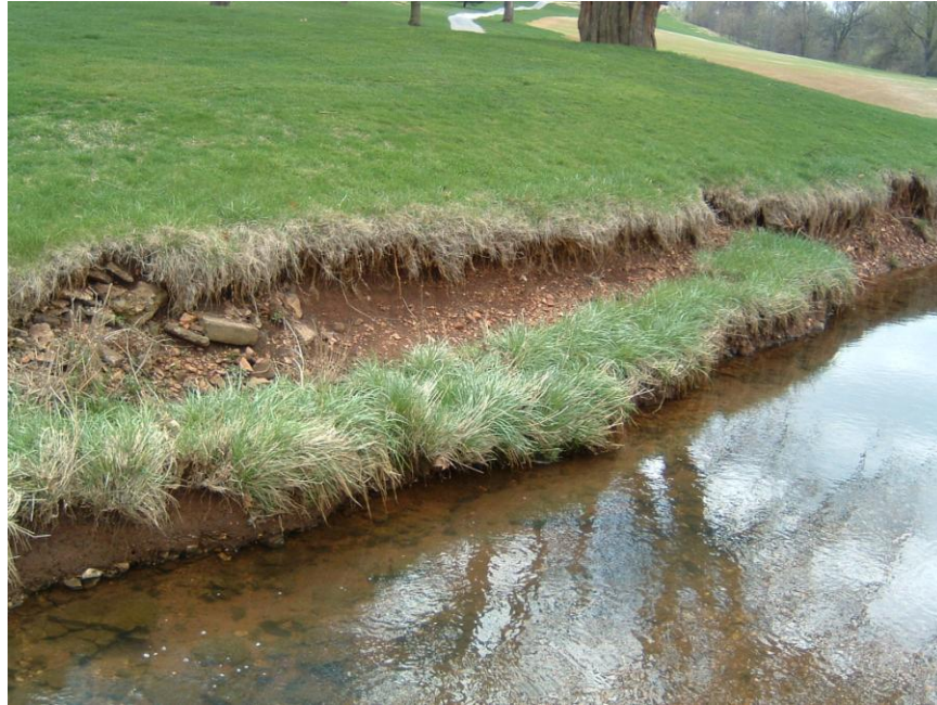
Photo 7. Bank failure due to poor riparian conditions in golf course reach
