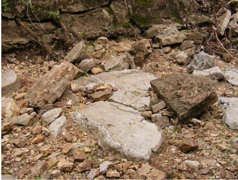
Photo 30. Large blocks from failing walls and construction rubble at station 500 feet SR-1 (4/6/09)
