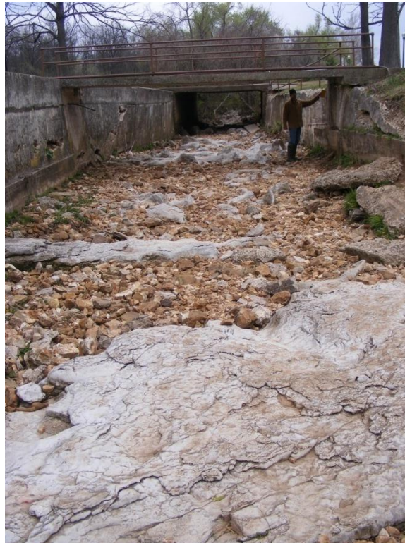
Photo 27. Bedrock bed near station 1,000 feet looking downstream SR-2 (4/6/09)
