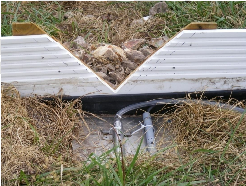
Photo 8. Pressure Transducer and Strainer Location
