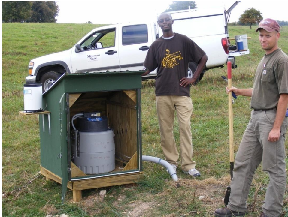
Photo 11. Auto-sampler and Rain Gage Installation (October 2008)
