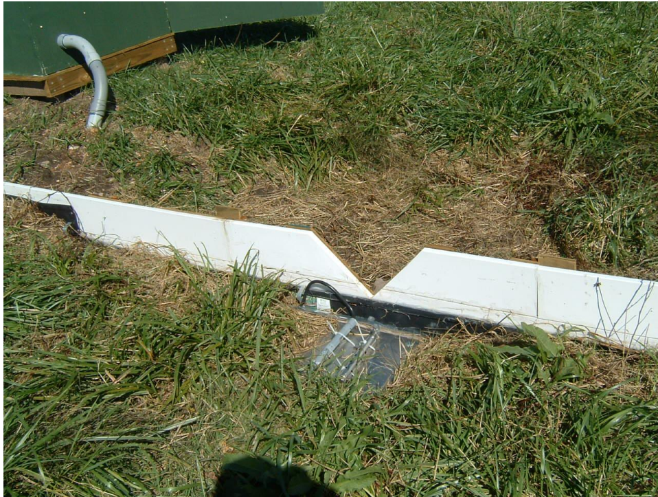
Photo 7. V-Notch Weir, Pressure Transducer, and Strainer Location
