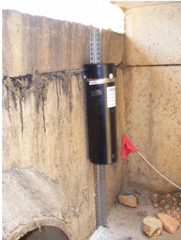
Photo 10. Curb inlet sampler installed at Park Hill
