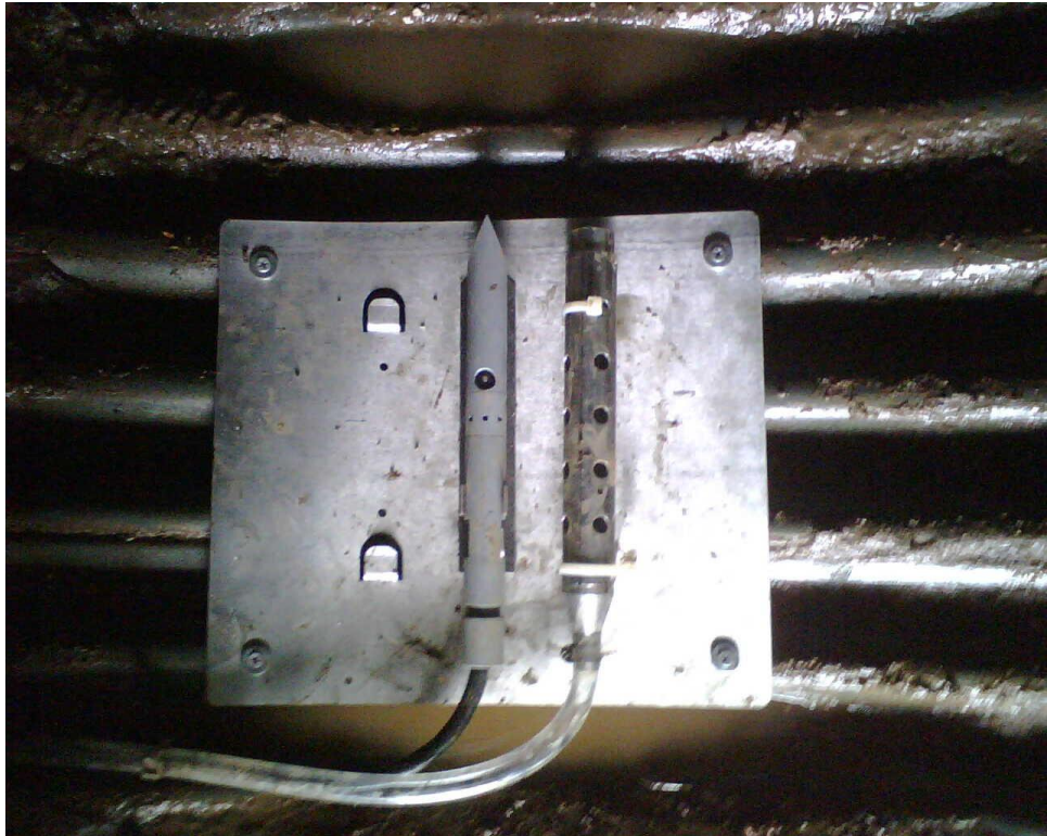
Photo 6. Mounted Pressure Transducer and Strainer in Pipe Invert
