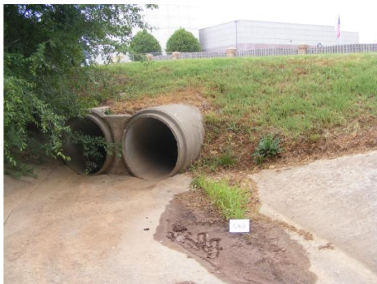
Sample 40- bed sediment accumulate at culvert outlet
