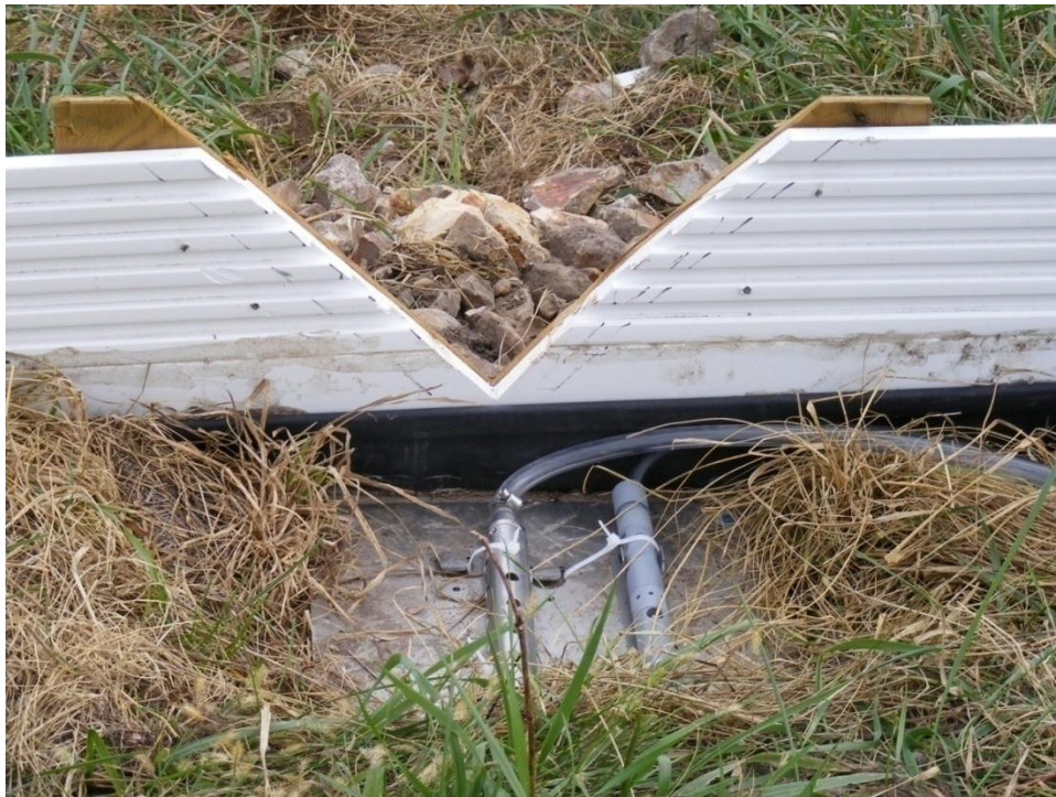
Photo 8. Pressure transducer and strainer location
