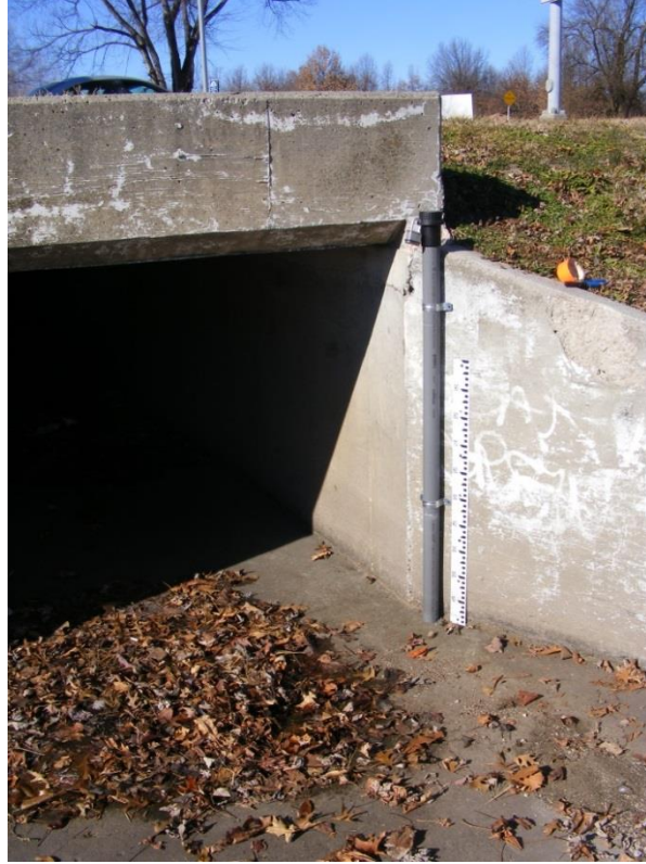
Photo 5. Levellogger housing and stage gage installed at National Avenue.
