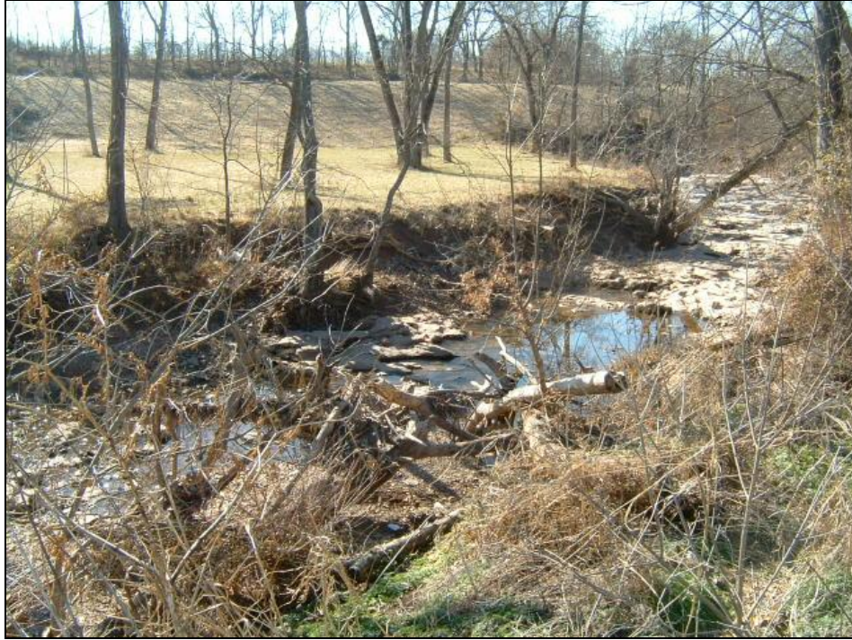
Figure 2.7: WC-above SWTP (2). Site at County Road 156 near Springfield, Missouri (February 5, 2006)
