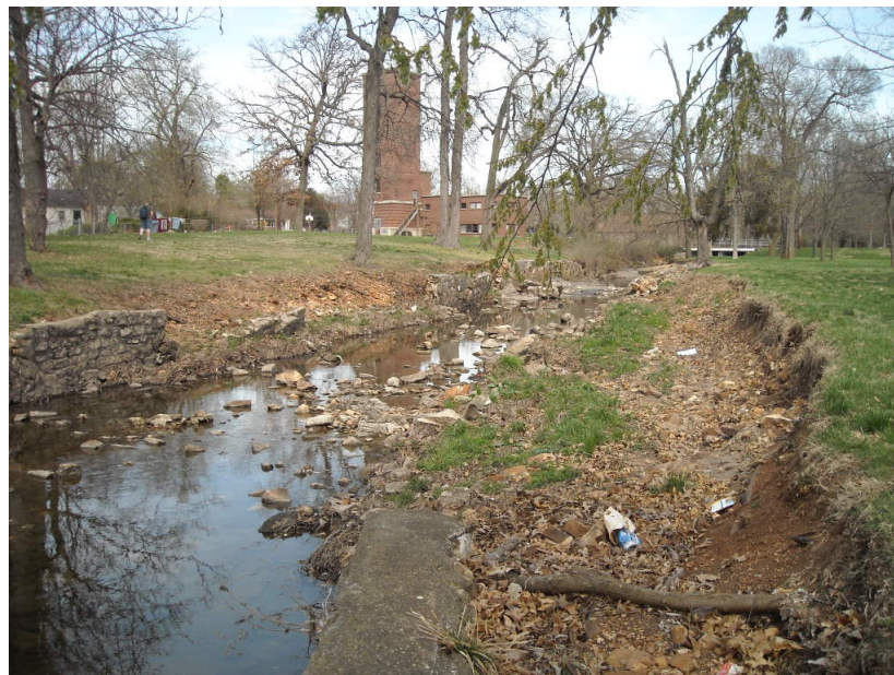
Figure 3. Channel erosion and widening in Fasnicht Creek in Springfield.
