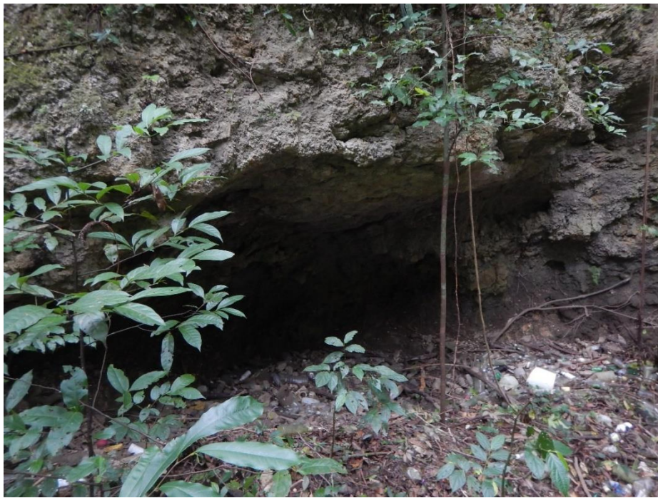
Appendix B-20. Point 17 – A “Scour Cave” on the Wall of the Brighton-Blue Hole Gorge Is an Erosional Feature Which Indicates the Removal of Wall Material Along Fractures
