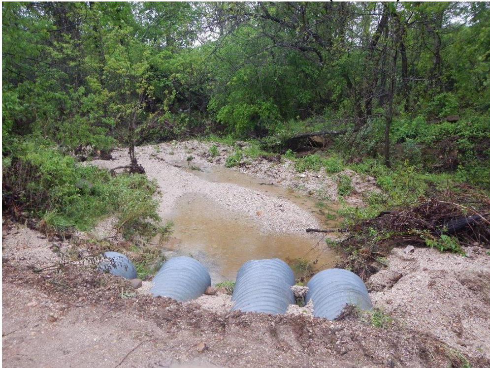
After Flood: Downstream View (5-4-2017)
