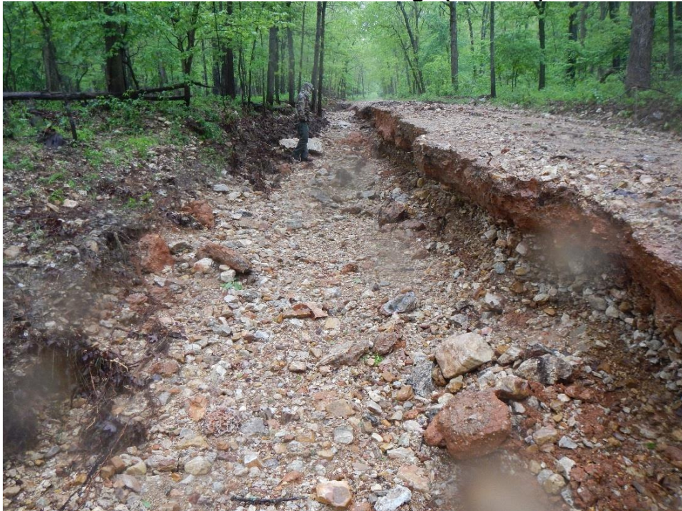
After Flood: Left Road Edge (5-4-2017)
