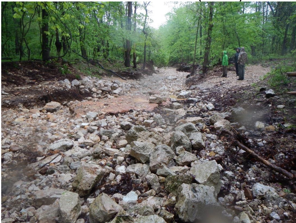
After Flood: Downstream View (5-4-2017)
