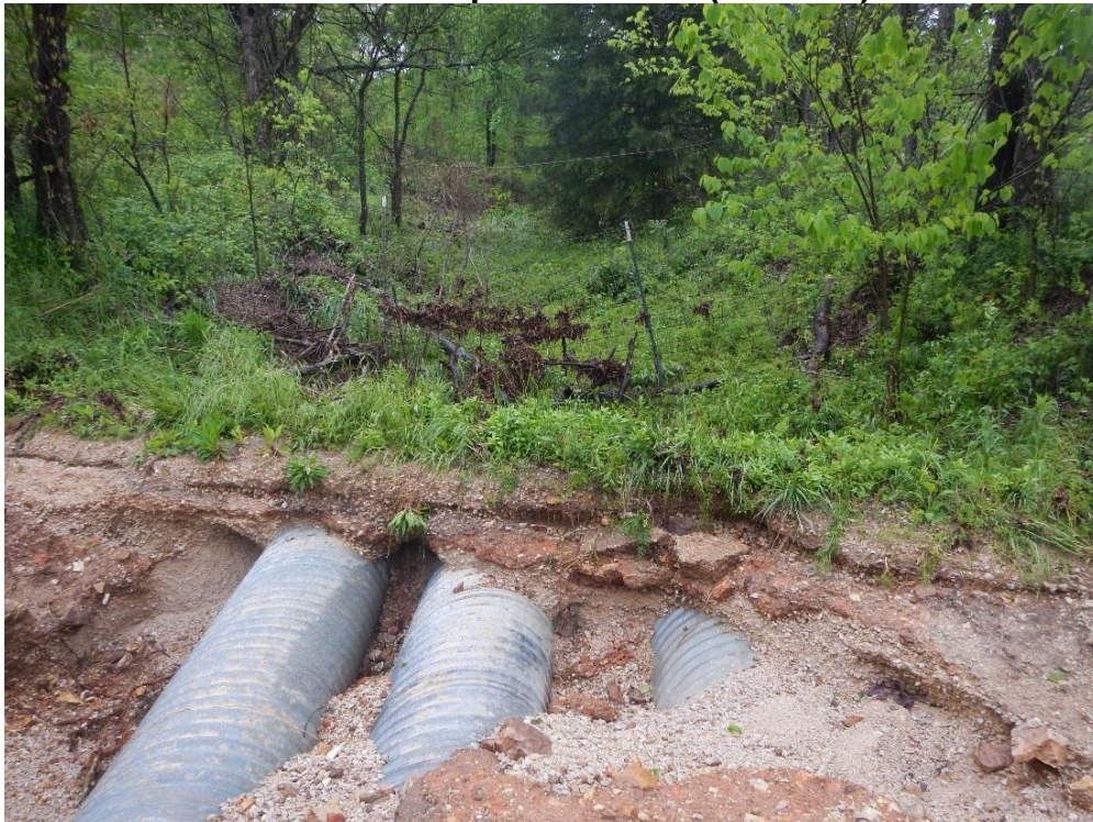
After Flood: Upstream View (5-4-2017)
