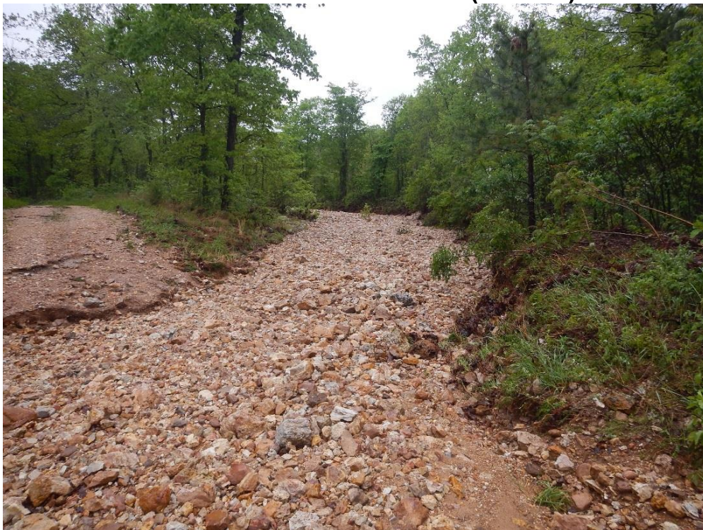
After Flood: Downstream View (5-4-2017)
