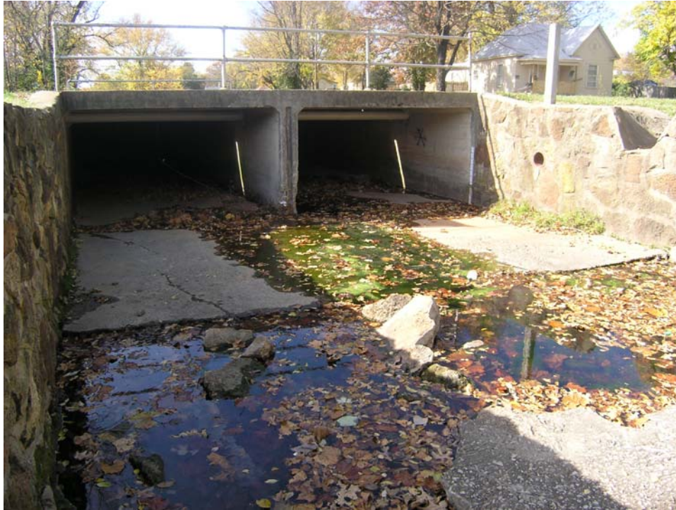
Site NB1 (North Branch Jordan at Fremont Ave): Downstream view showing gage location, dry channel and karst seep
