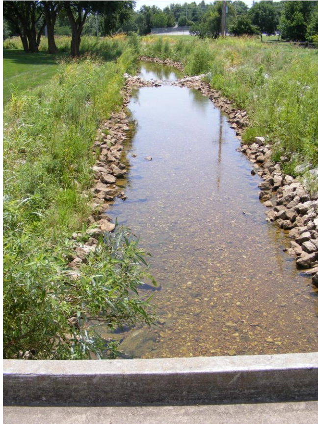
Picture 23. Vegetation growth in composite revetment, July 2008 (St. 750 ft)
