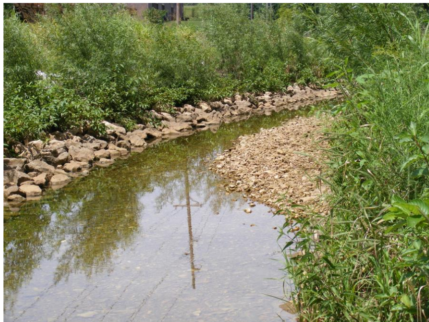
Picture 24. Gravel bar formation at bankfull bench, July 2008 (St. 950 ft)
