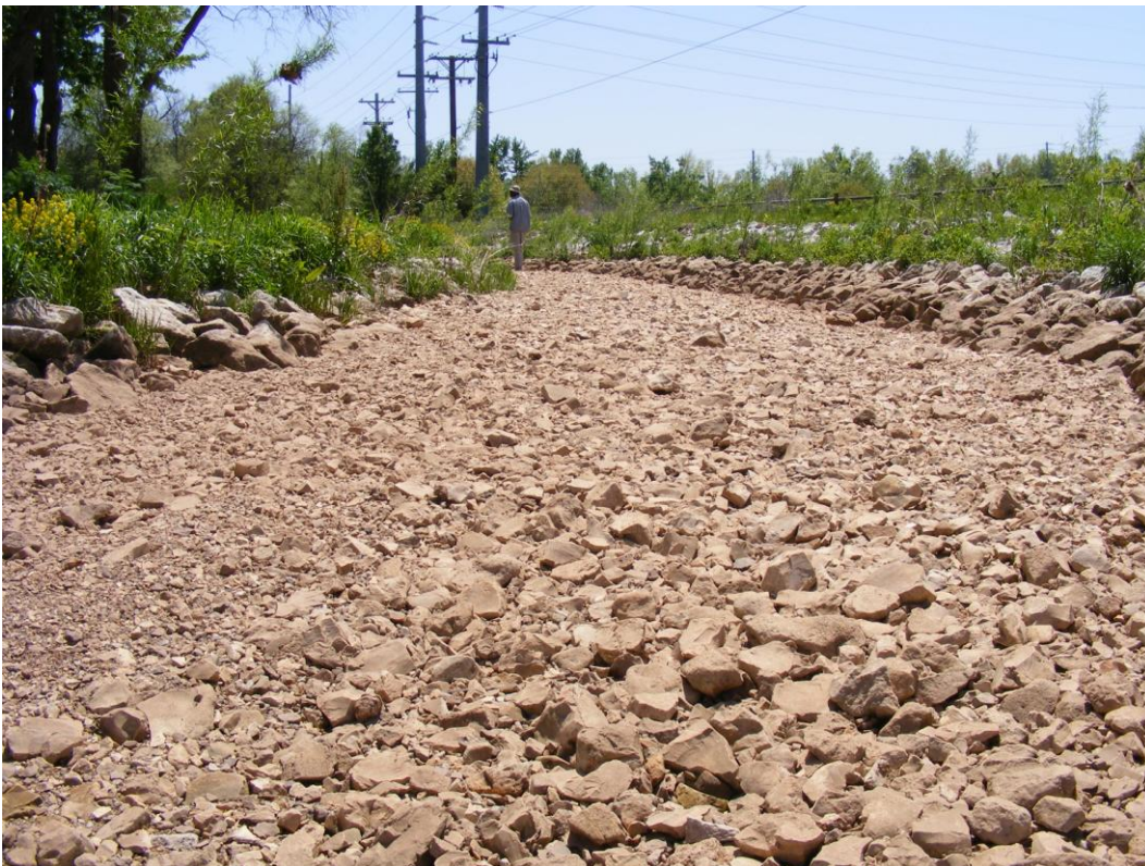
Picture 18. AFTER - Composite revetment installed on high west bank looking downstream May 2008 (St. 1,000 feet)
