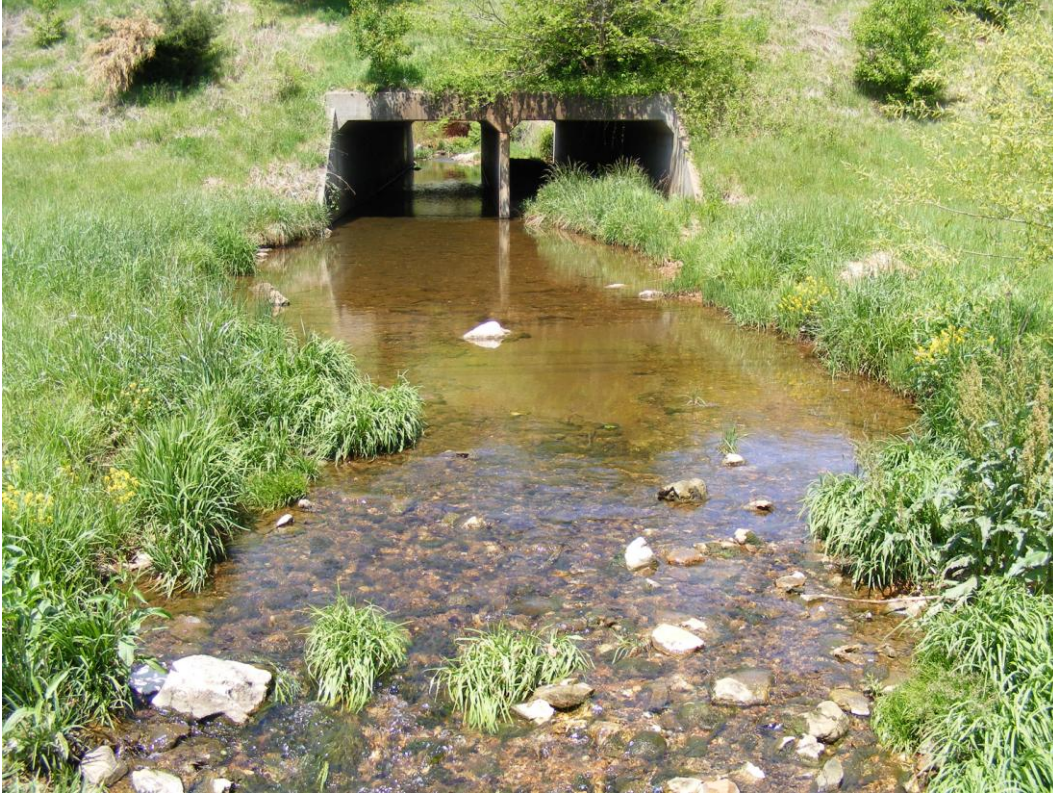
Picture 1. Republic Road bridge upstream of upper cart bridge looking upstream May 2008 (St. 100 feet)
