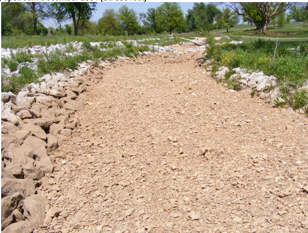
Picture 14. AFTER - Maintained riffle crest position, bank protection and enhanced riparian corridor May 2008 (St. 900 feet)
