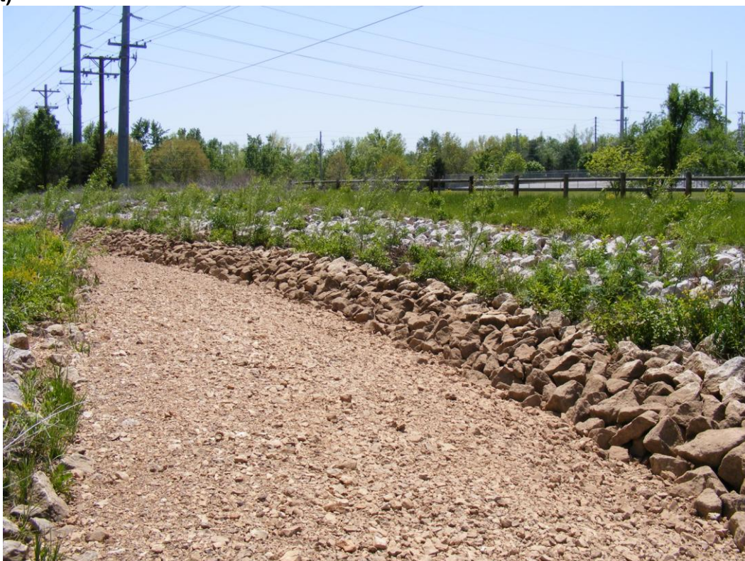
Picture 6. Composite revetment along the once active eroding reach looking downstream May 2008 (St. 1,000 feet)
