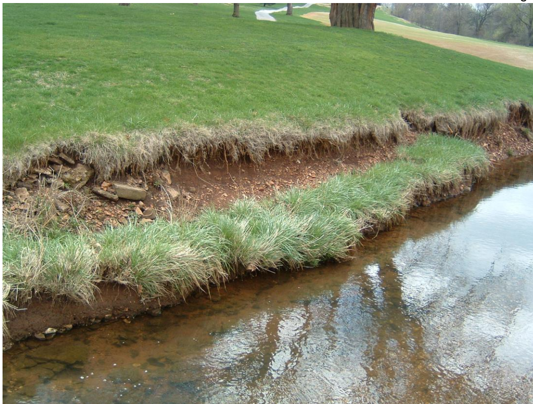
Picture 15. BEFORE - High bank angle collapse above second cart bridge looking downstream August 2005 (St. 700 feet)
