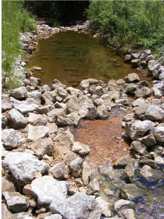
Picture 25. Undermined grade control structure exposing residuum, July 2008 (St. 1,120 ft)
