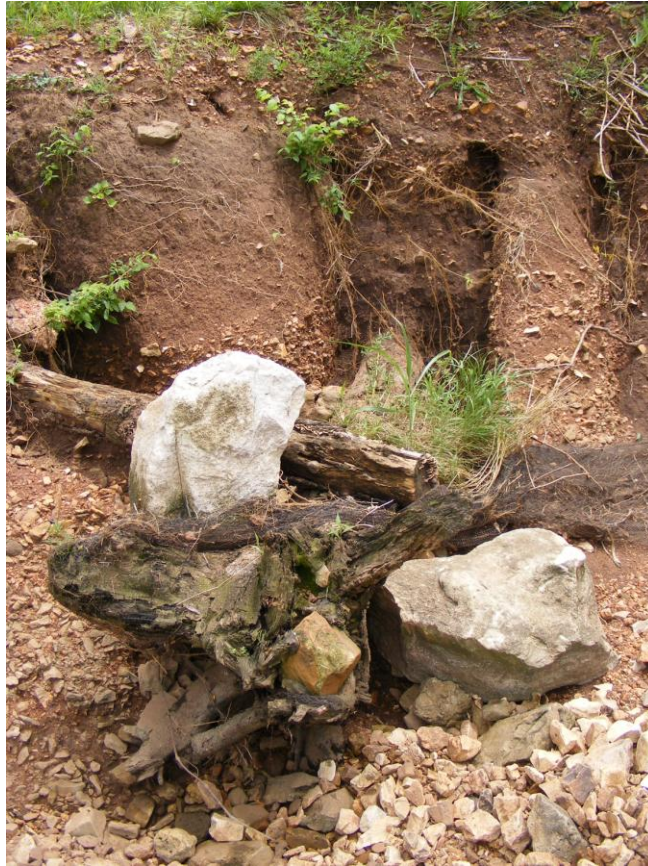
Picture 29. Bank failing at backfilled trench behind root wads, July 2008 (St. 1,660 ft)
