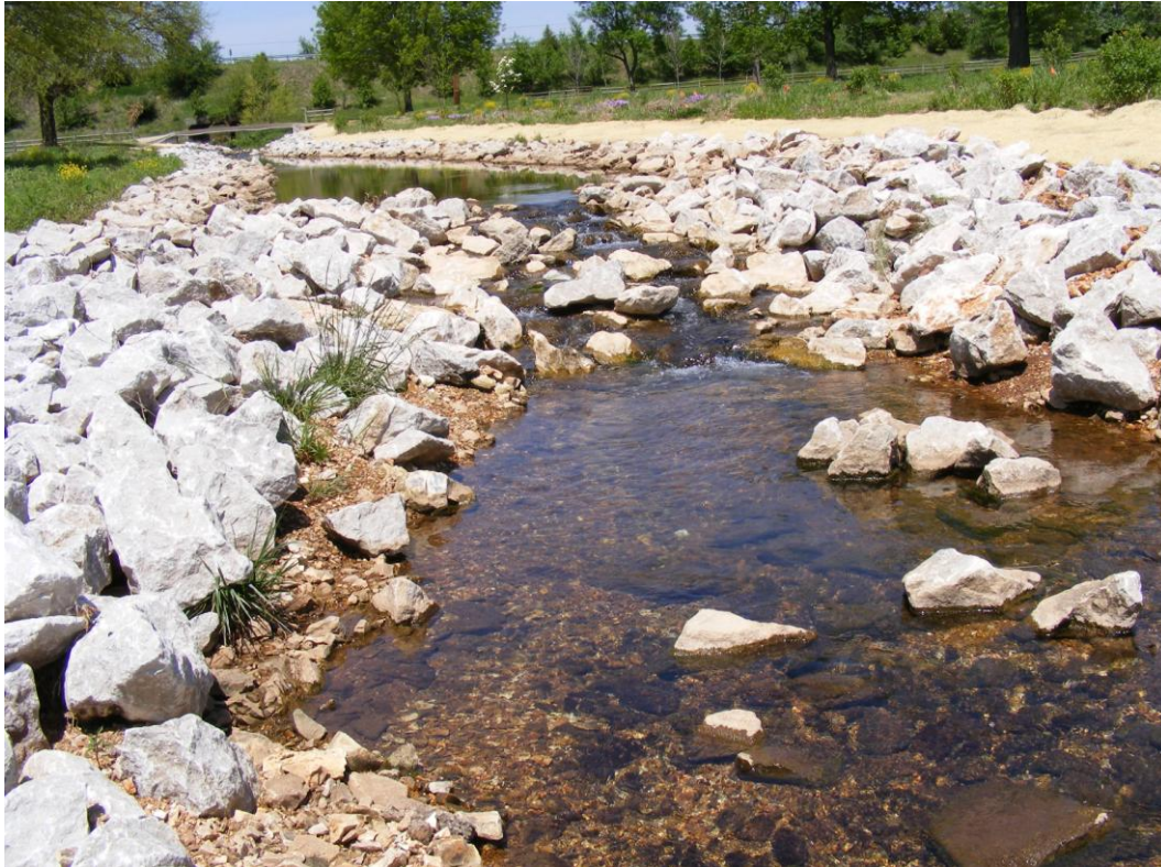
Picture 3. Example of grade control structure downstream of upper cart bridge looking upstream May 2008 (St. 450 feet)
