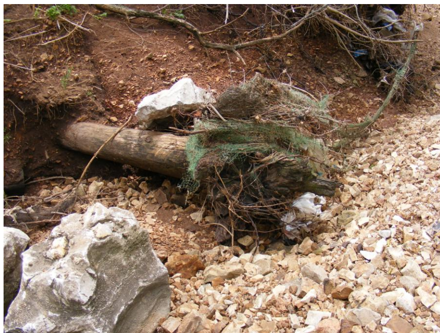
Picture 30. Missing header log at root wad structure, July 2008 (St. 1,660 ft)
