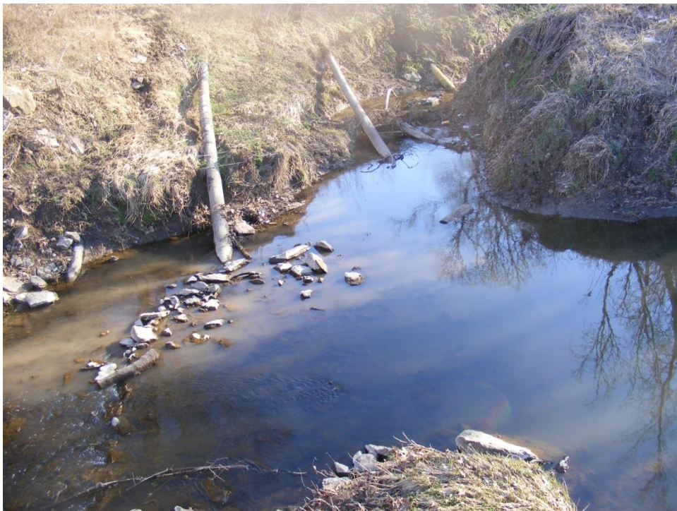
Photo 6. Example of problem type 6. Exposed pipes or cables due to erosion
