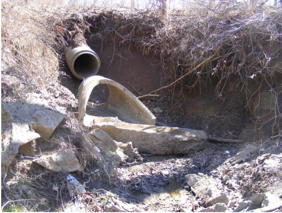
Photo 7. Example of problem type 7. Failed culvert/inlet due to undermining
