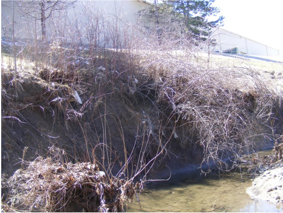
Photo 1. Example of problem type 1. Bank erosion and failure risk-commercial property
