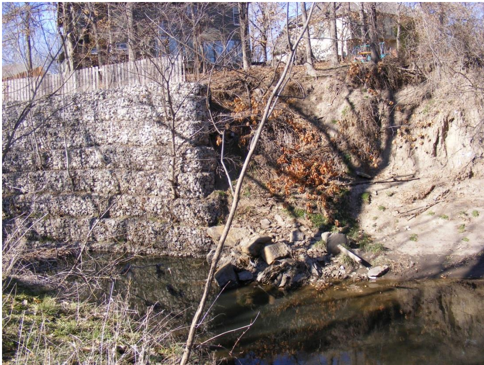
Photo 4. Example of problem type 4. Bank erosion and failure risk-residential private
