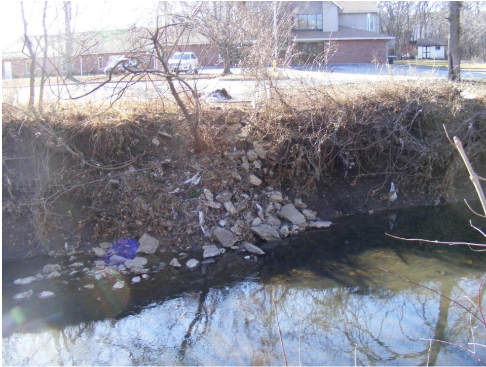
Photo 3. Example of problem type 3. Bank erosion and failure risk-public building
