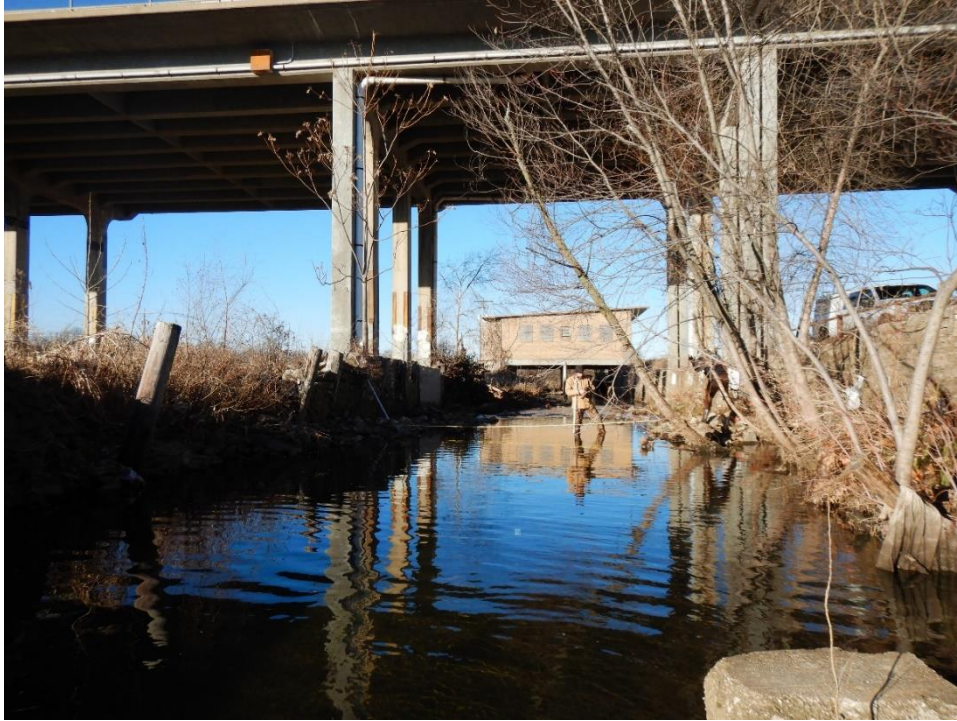
Photo 3. Grant Ave Bridge located 663 feet downstream of the underground looking upstream. (Photo taken January 25, 2019)
