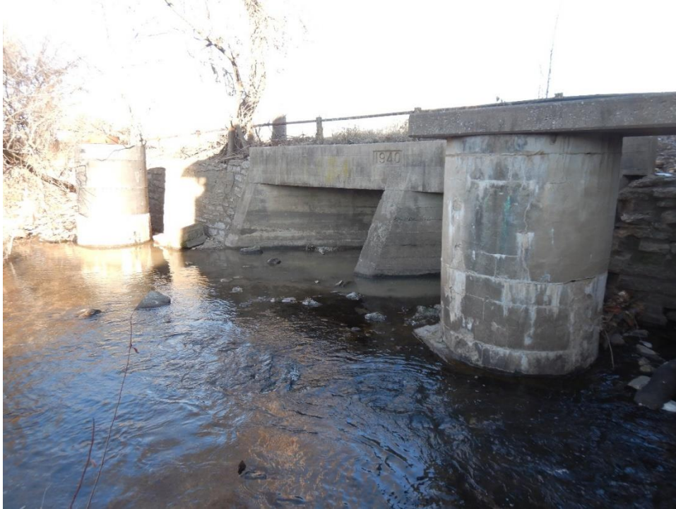
Photo 1. Two sewer manholes and a large culvert located at 876 feet downstream of the underground along the north bank. (Photo taken January 25, 2019)
