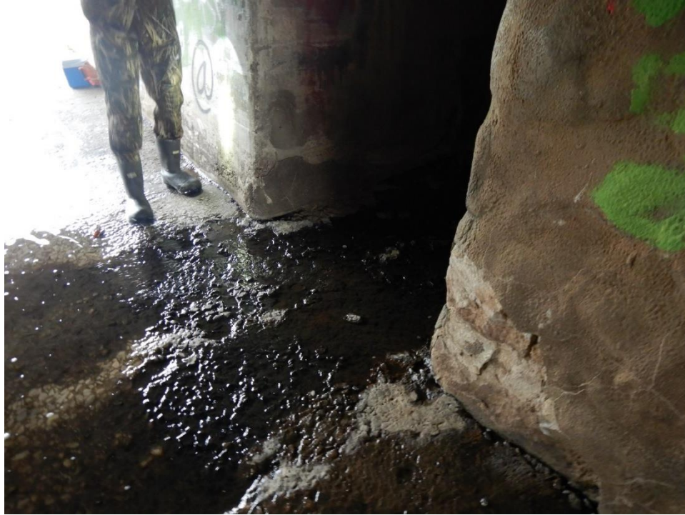
Photo 5. Storm drain under Main Ave Bridge 100 ft downstream of the underground along north bank. (Photo taken January 25, 2019)
