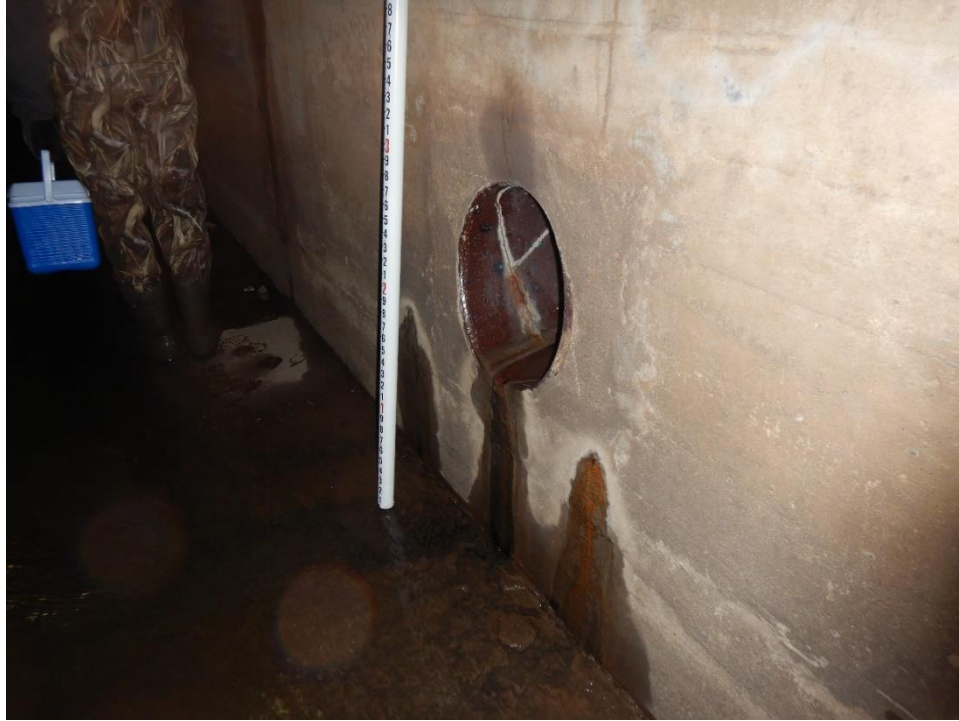
Photo 9. Large drain pipe at 2,200 feet along the north exterior wall of the north culvert. (Photo taken January 25, 2019)
