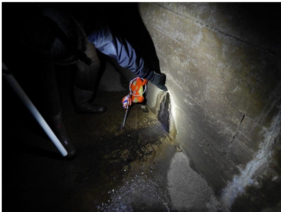
Photo 10. Seep at 2,500 feet on the exterior wall of the north culvert. These types of seeps are common throughout the underground. (Photo taken January 25, 2019)
