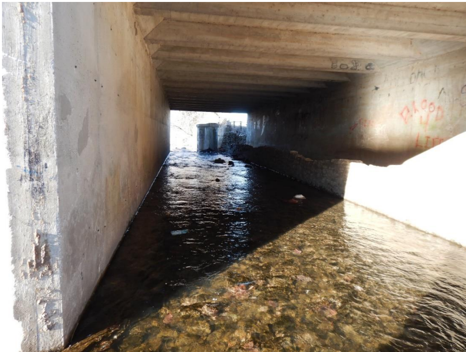
Photo 2. Building over creek located 816 feet downstream of the underground looking upstream. (Photo taken January 25, 2019)
