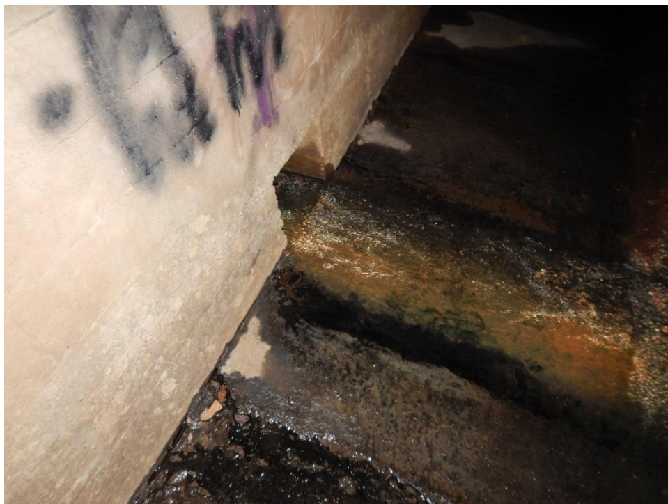
Photo 6. Larger drain at 800 ft in the south culvert along south exterior wall. Several other drains and seeps enter the south culvert downstream of Campbell Ave. (Photo taken January 25, 2019)
