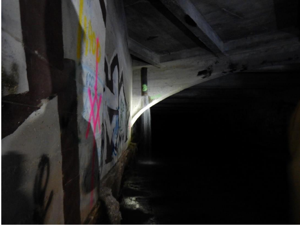
Photo 7. Sump pump at 1,380 feet in the combined culvert on the south side. (Photo taken January 25, 2019)
