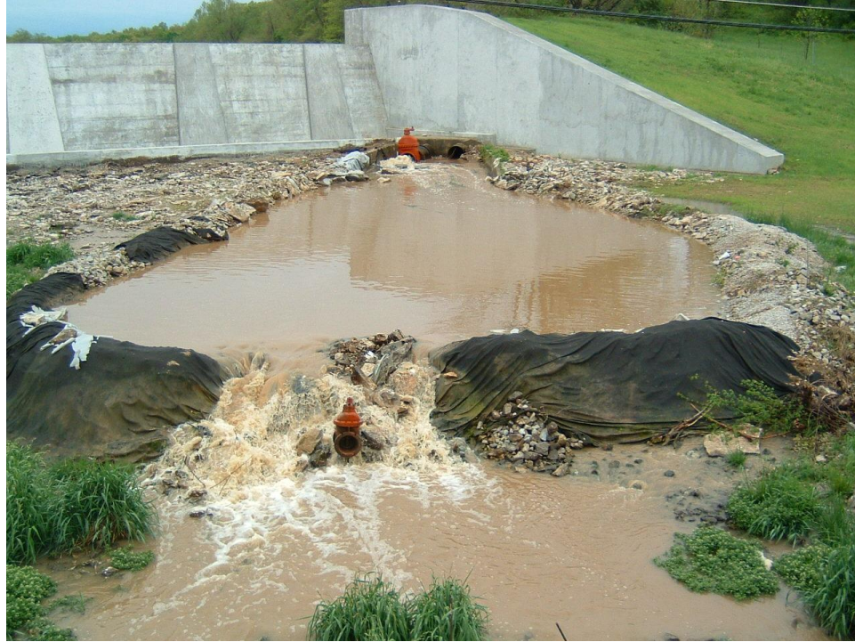
Figure 3.5 Detention Pond and Drainage Valve Located at the Base of the Valley Mill Reservoir Spillway
