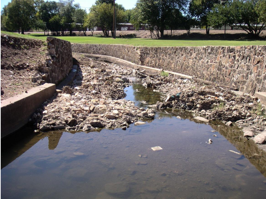
Figure 31. Failed bank armoring along Jordan Creek upstream of site 39. Photo by D.J. Wurglitsh. Used with permission.
