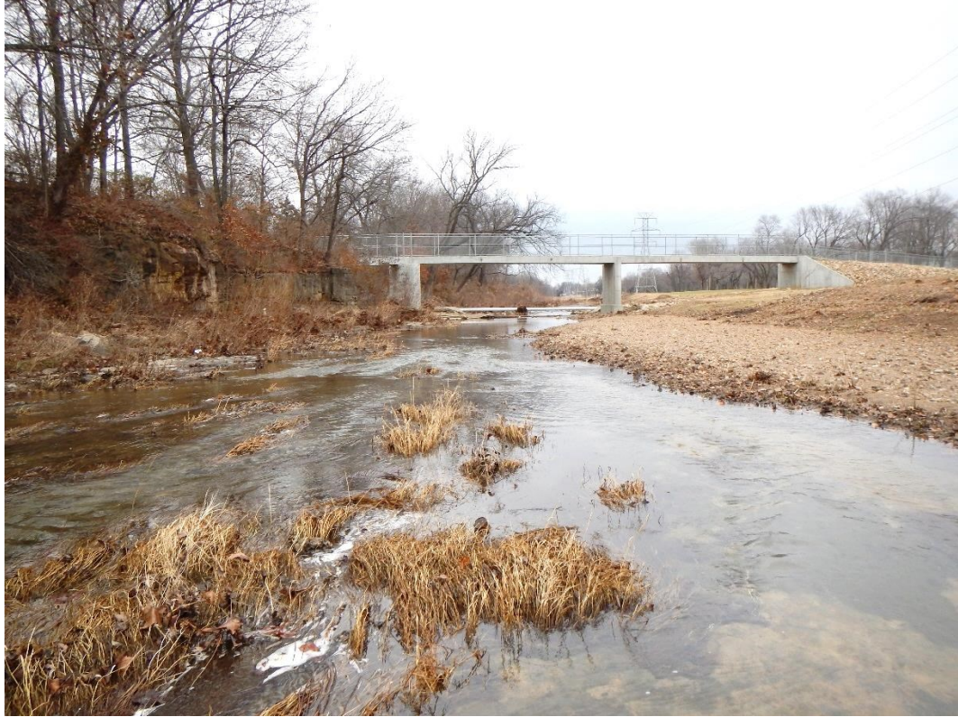
Active bar deposits and steep channel banks at R-km 5.8.
