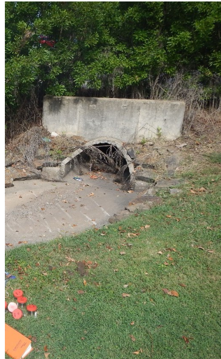
Fig. 18. Trickle channel leading to Central outlet (A). Trickle channel located in West sub-basin (B)
