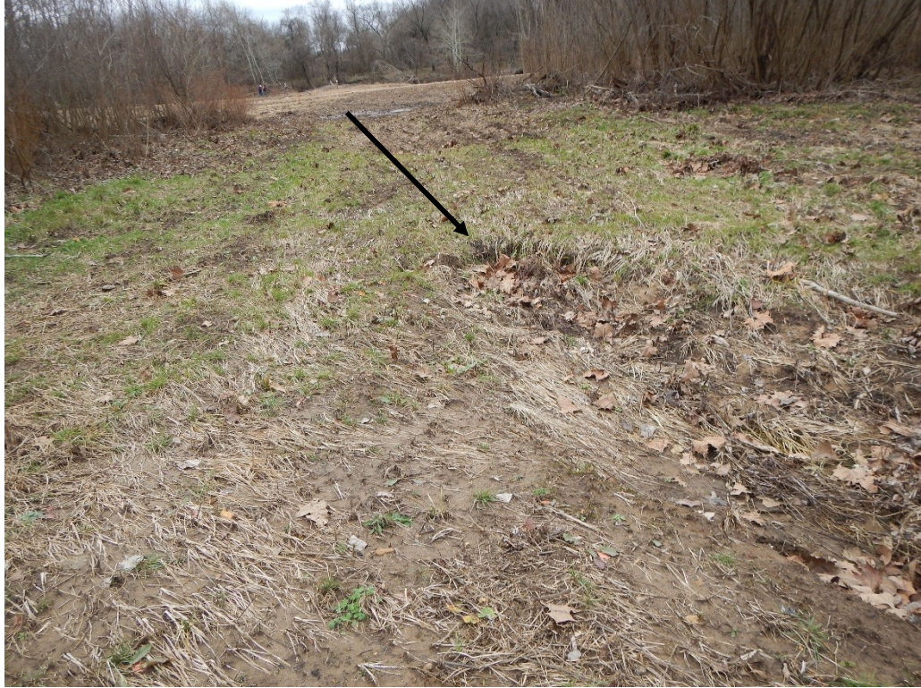
Headcut within well-drained flood way looking back towards the upper basin (12/14/15).
