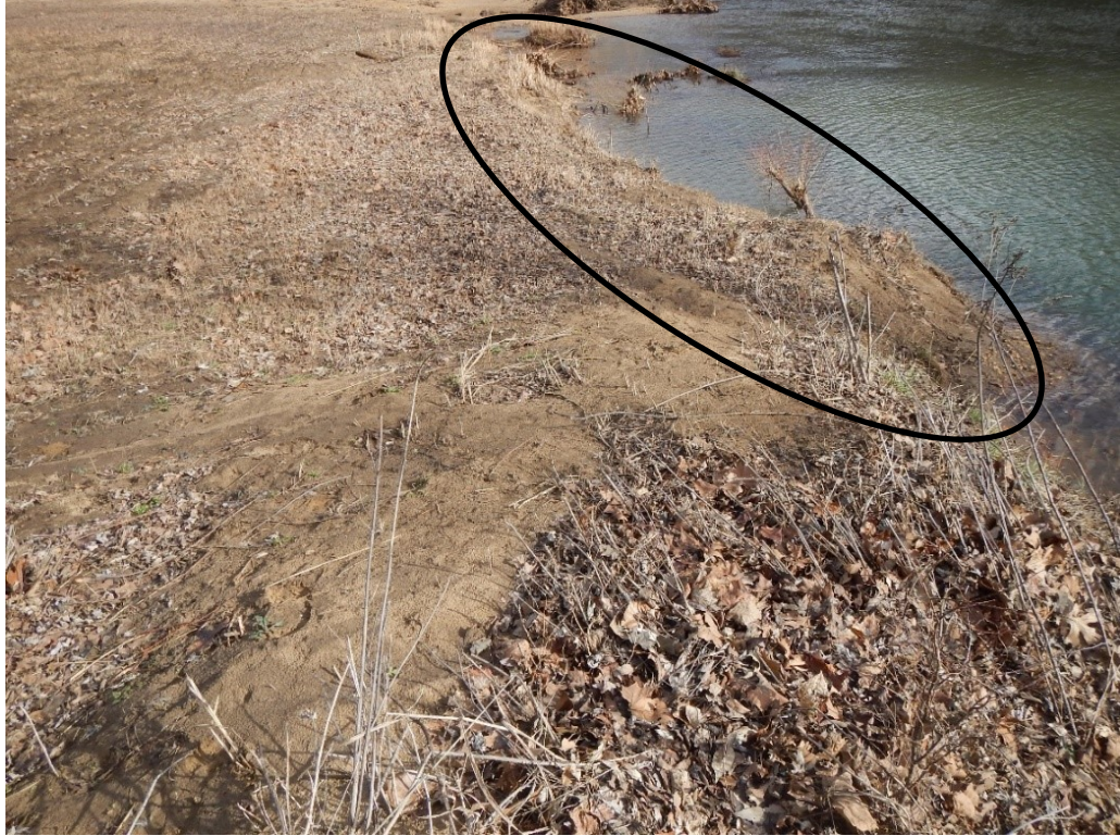
Figure 24. Bank erosion along bank of upper basin (12/14/15).
