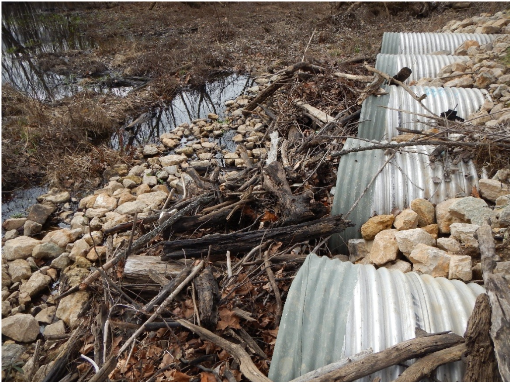
Debris jam blocking primary outlet (12/14/15).
