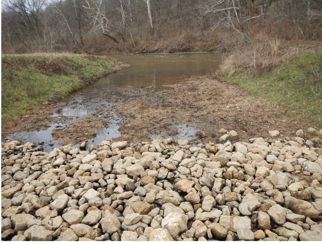
Primary outlet to Big River from culverts (12/14/15).
