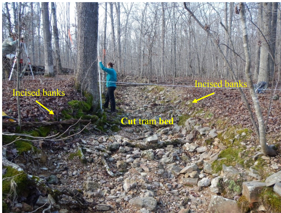
Figure 13. Tram Bed Forced Morphology Photos. A) Incised channel along filled tram bed, R-km 1.17, B) Incised channel in cut tram bed, R-km 0.93. Photos taken Dec. 2015.
