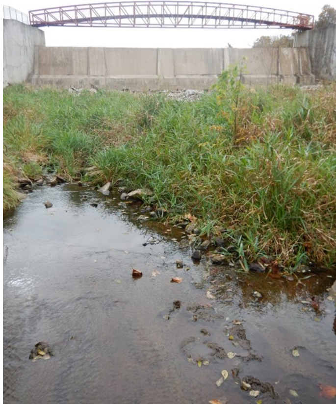
Figure 16. Valley Water Mill Reservoir seepage
