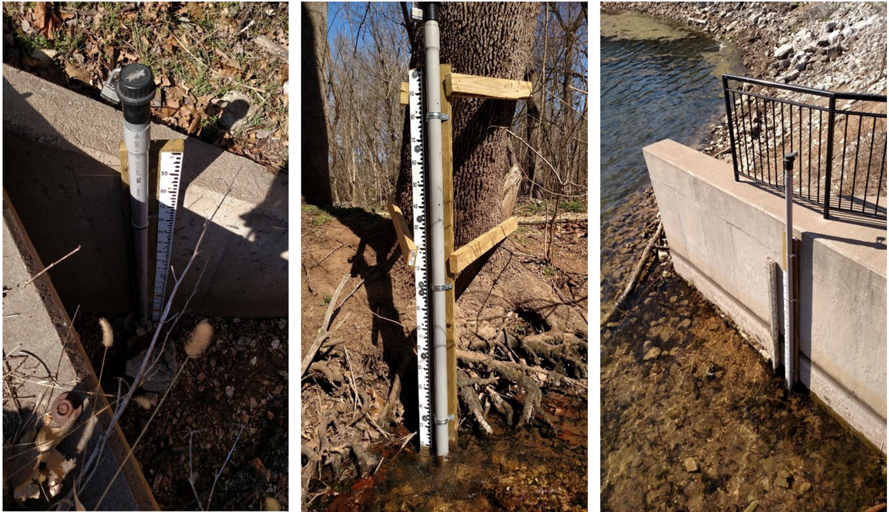
Figure 19. Continuous stage gages installed at sites FR-102, SS2, and RD
