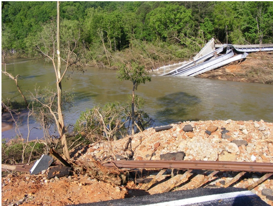
Figure 56. Deck of the Highway CC Bridge that was destroyed during the April Flood.
