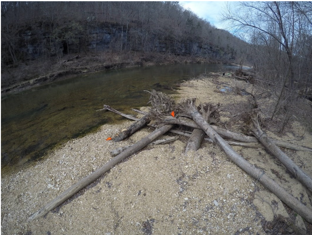
Figure 10. ELS 4 in foreground and ELS 3 in background. Flow direction from right to left and burial of key pieces with root fans oriented upstream.
