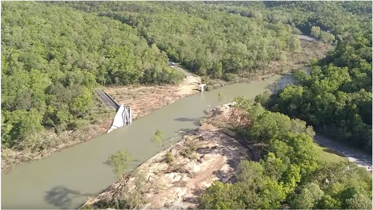
Figure 23. Highway CC bridge at NFRA. Deck of bridge washed downstream of road. (Aerial Ozarks, 2017).
