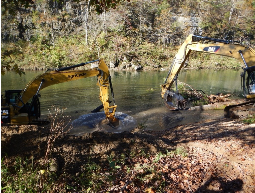
Figure 5. Construction of ELS 1. Excavator digging a trench in the bed for key piece placement.
