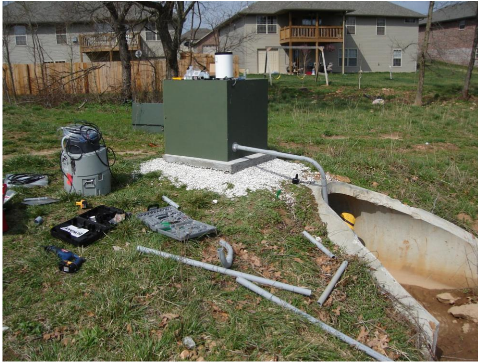
Figure 1. Monitoring Station and Sampler Installation. Monitoring station has been installed on a concrete slab above the pipe outlet.
