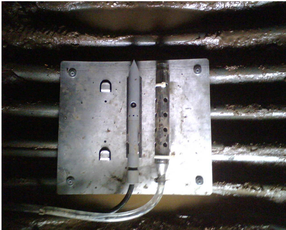
Figure 2. Pressure Transducer and Strainer Installation. Mounting plate with pressure transducer and sample tubing intake installed in the invert of a corrugated metal pipe.
