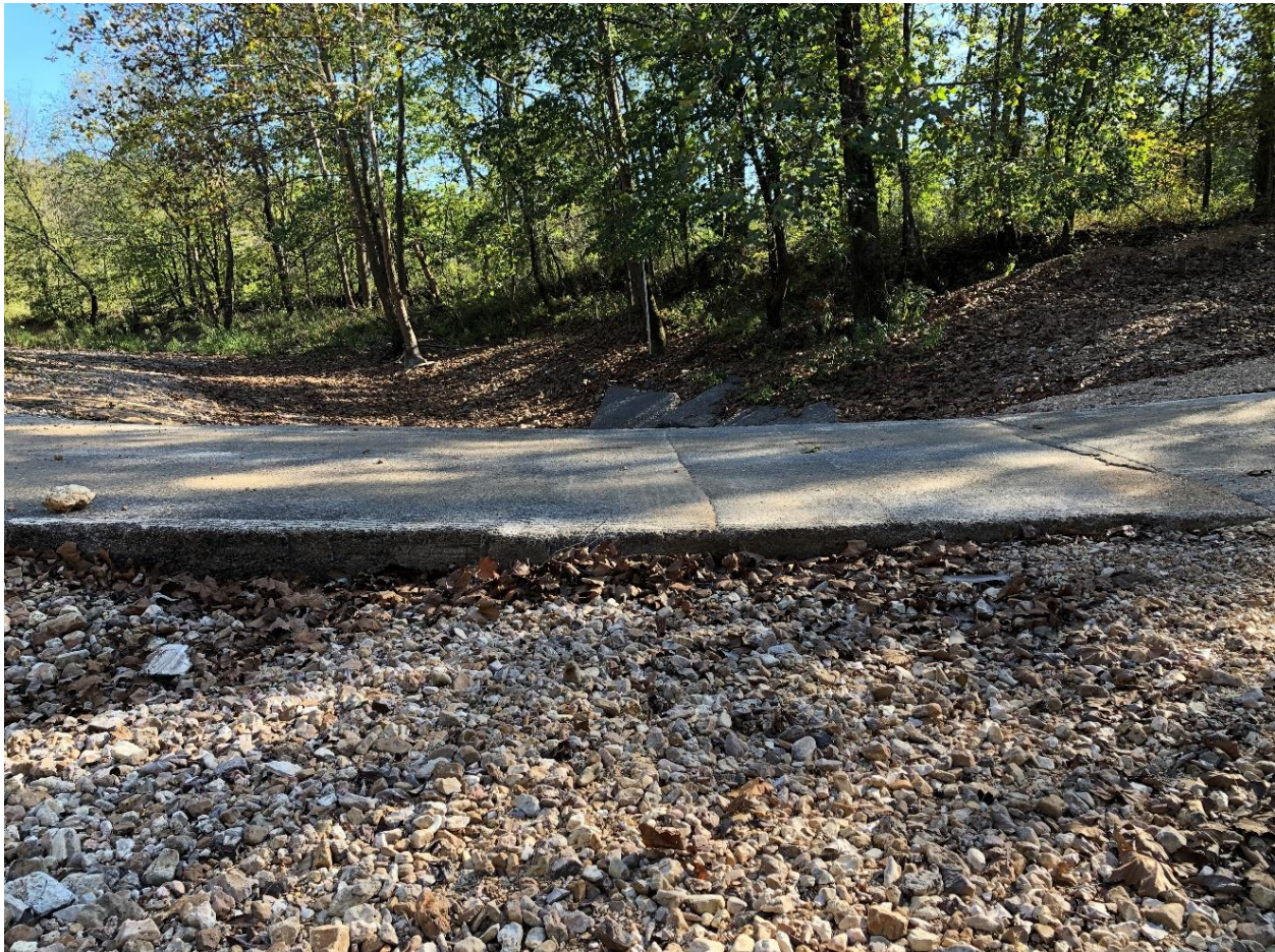
Photo 20. Gage at LBB looking downstream of low water crossing at Ripley County C-10 (Oct 22, 2019).
