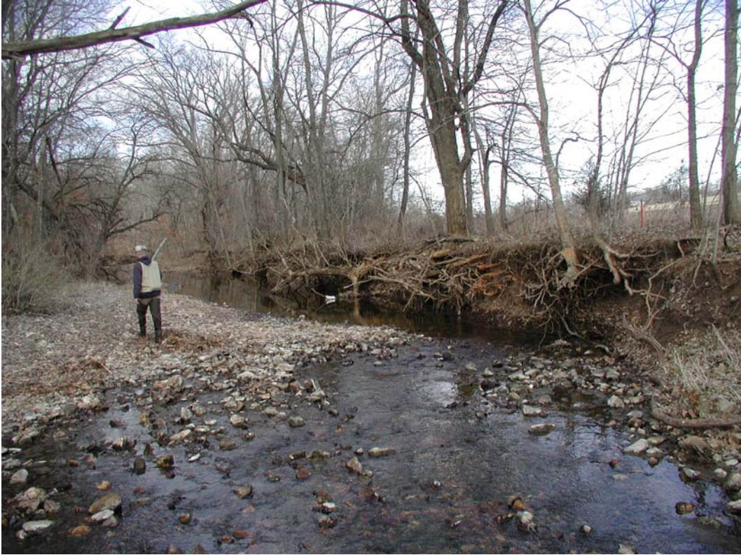
Picture 11. Exposed roots along eroding bank looking downstream (400 m)
