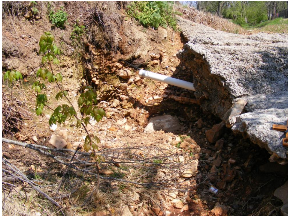
Picture 30 - Exposed phone line (4-29-08)
