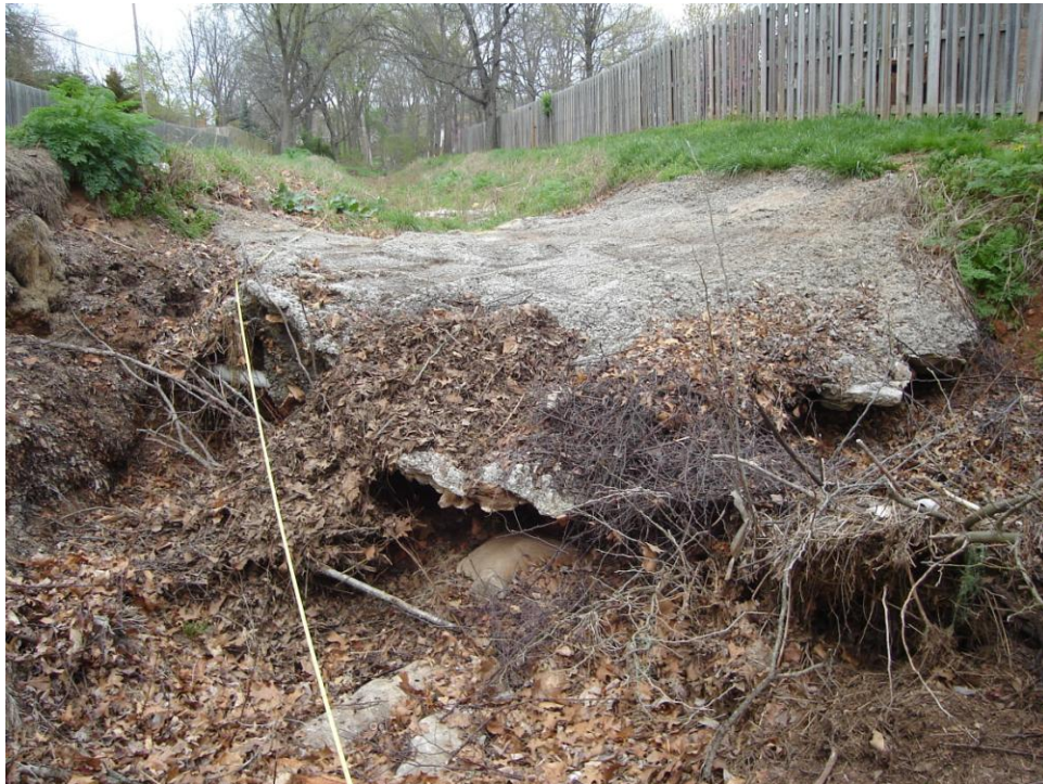
Picture 2 – Concrete bed obstruction/headcut at 670ft (looking upstream)
