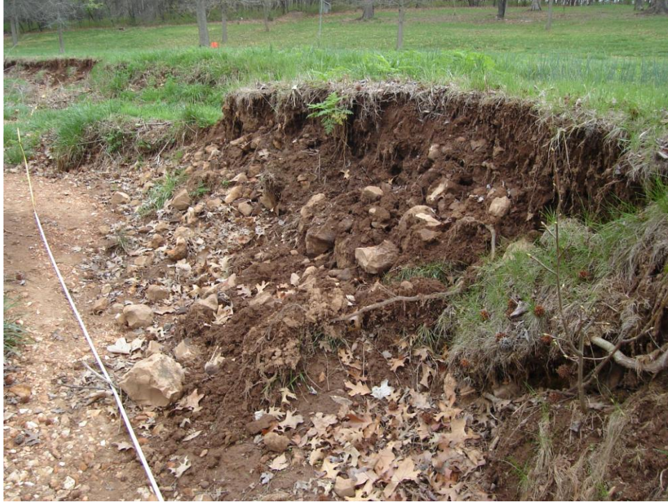
Picture 9 – Slumping, failing bank just above stream crossing at ~320ft (Sub-reach #4) Notice: Maybe old channel bed deposits collapsing into the present channel.
