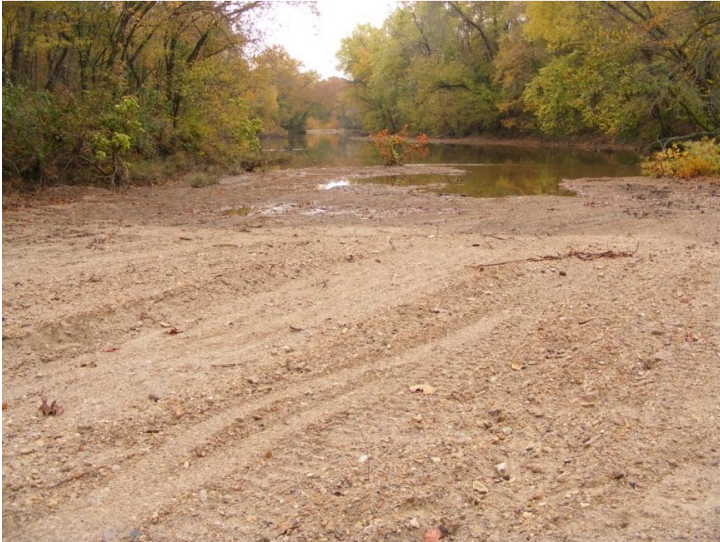
Looking upstream across excavated bar head. Notice excavator tracks and flat topography.
