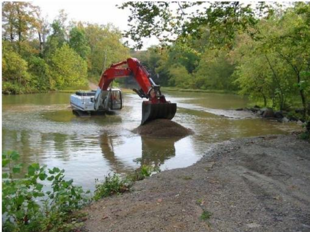
Excavation activities at the Bone Hole site are consistent with post-excavation survey results. (Photos from HGL Field Oversight Report).
