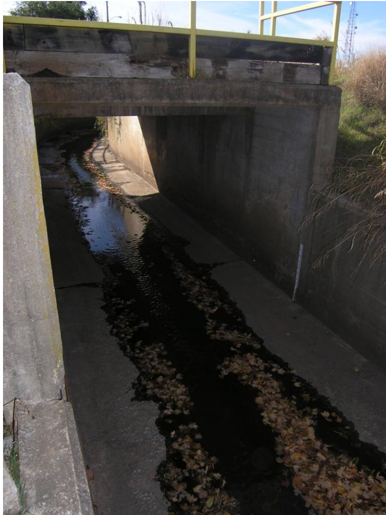
Site SB2 (South Branch Jordan at Hammons Parkway): Downstream view showing gage location and base flow. Base flow stream gaging was done at channel center and event stages were reported as staff gage reading plus elevation difference between gage base and channel center.
