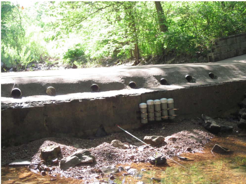
Figure 3.2 Downstream edge of the upstream low-water bridge Location 0 m on tapeline (April, 2012).
