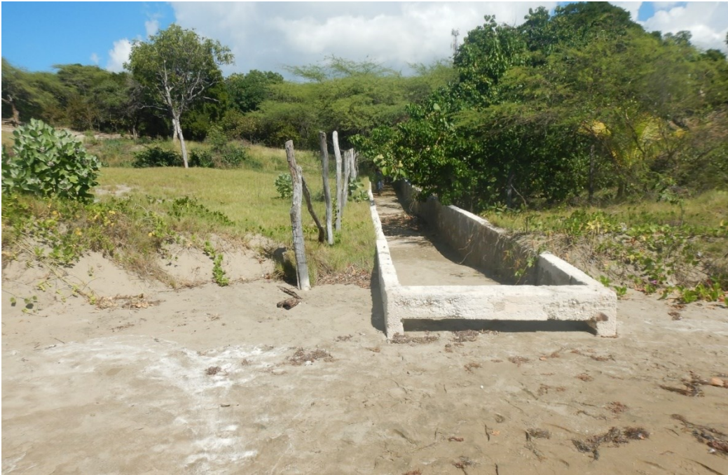
Waterway draining on the backbeach at Billy's Bay.
