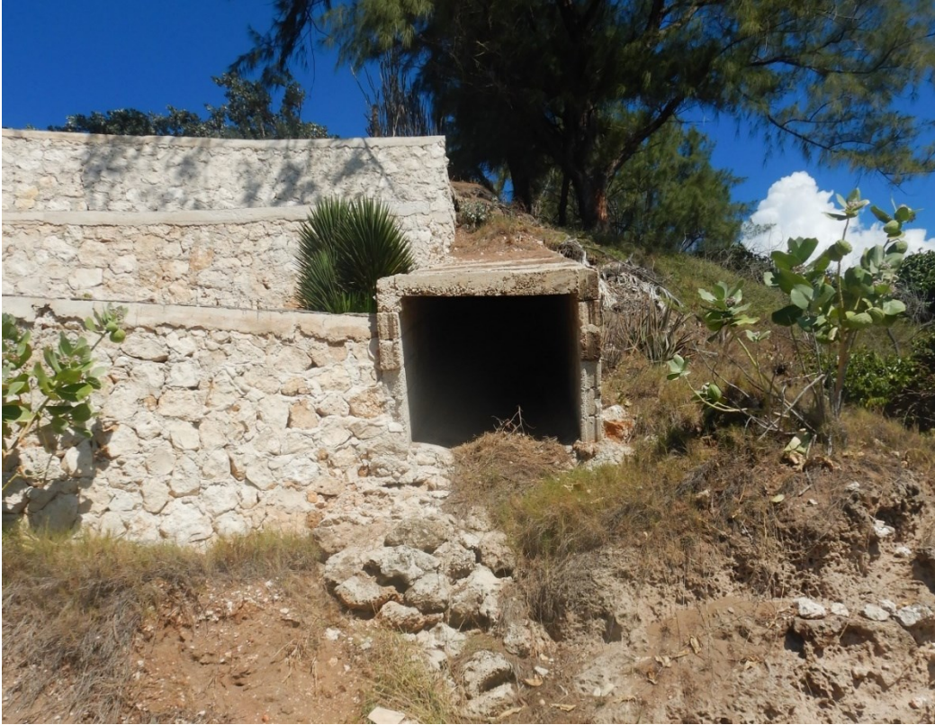
Drainage system draining on the beach at Billy's Bay.
