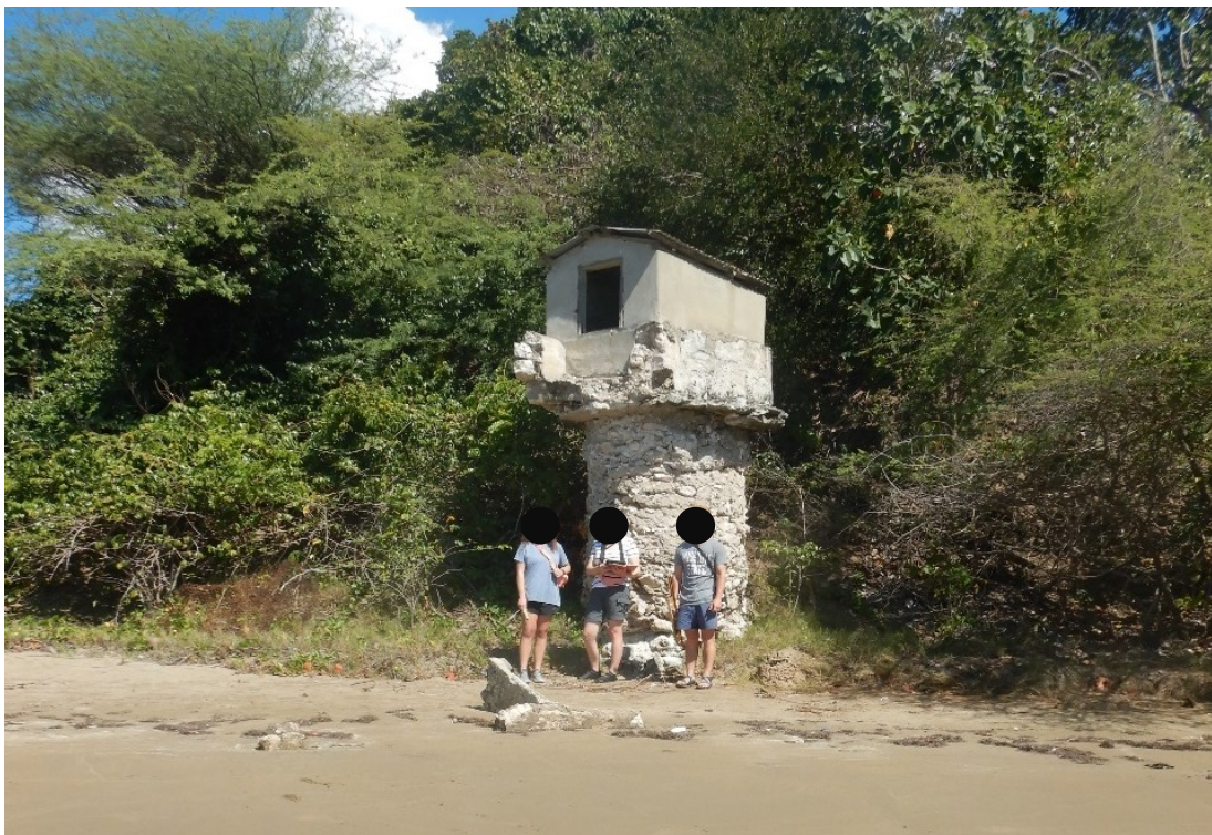
Figure 24. Example of an eroding beach, exposing a well house and pit wall at Billy's Bay (01/12/2021).
