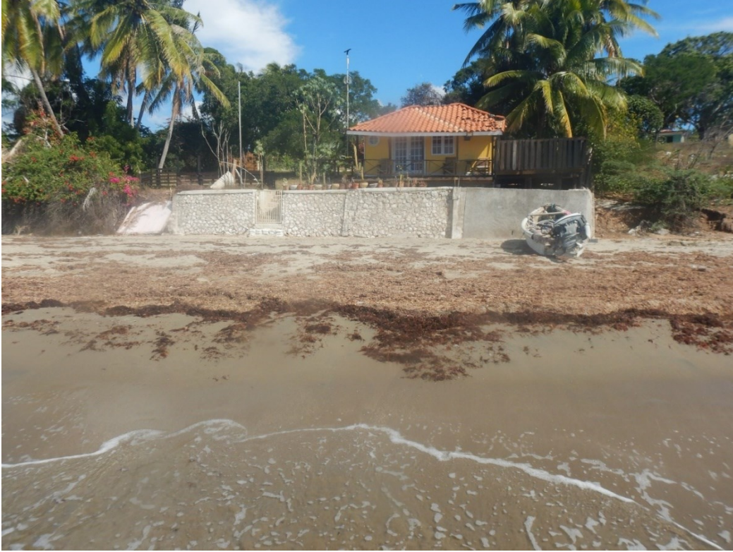
Narrow beach with cement and stone wall on the backbeach at Great Bay.
